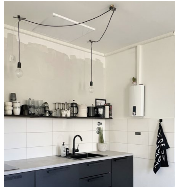
Ceiling heating in the kitchen.
